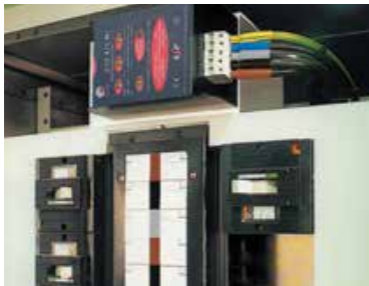
Figure 1: ESP 415 M1 installed inside a power distribution panel.
