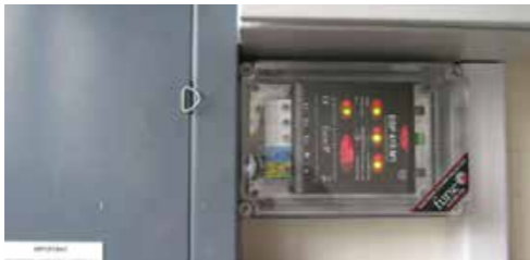
Figure 2: ESP 415 M1 installed next to a power distribution panel.
